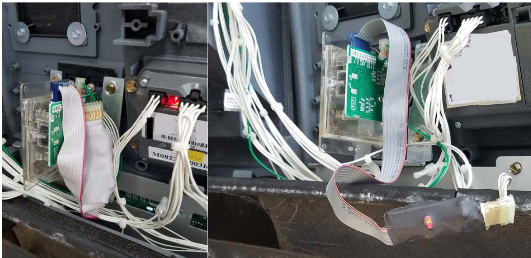
Skimming devices found on two pumps at the Kangaroo Express at 1201 Palm Harbor Parkway in Palm Coast.
